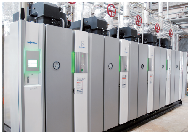
蒸気ボイラ(3t/h×5台)
